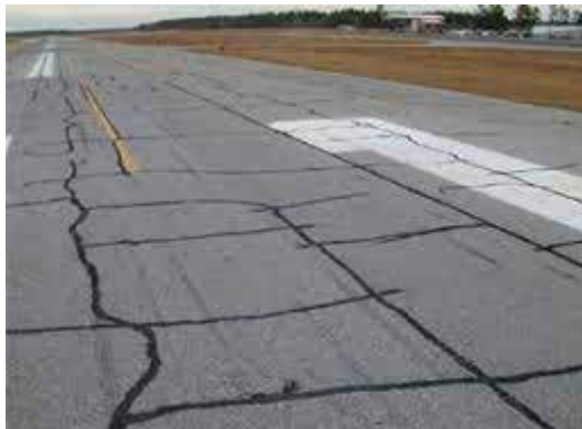
Weather-related box cracking
