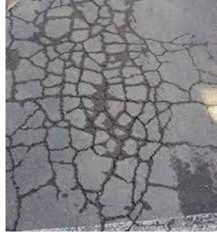
Structural-related alligator cracking
